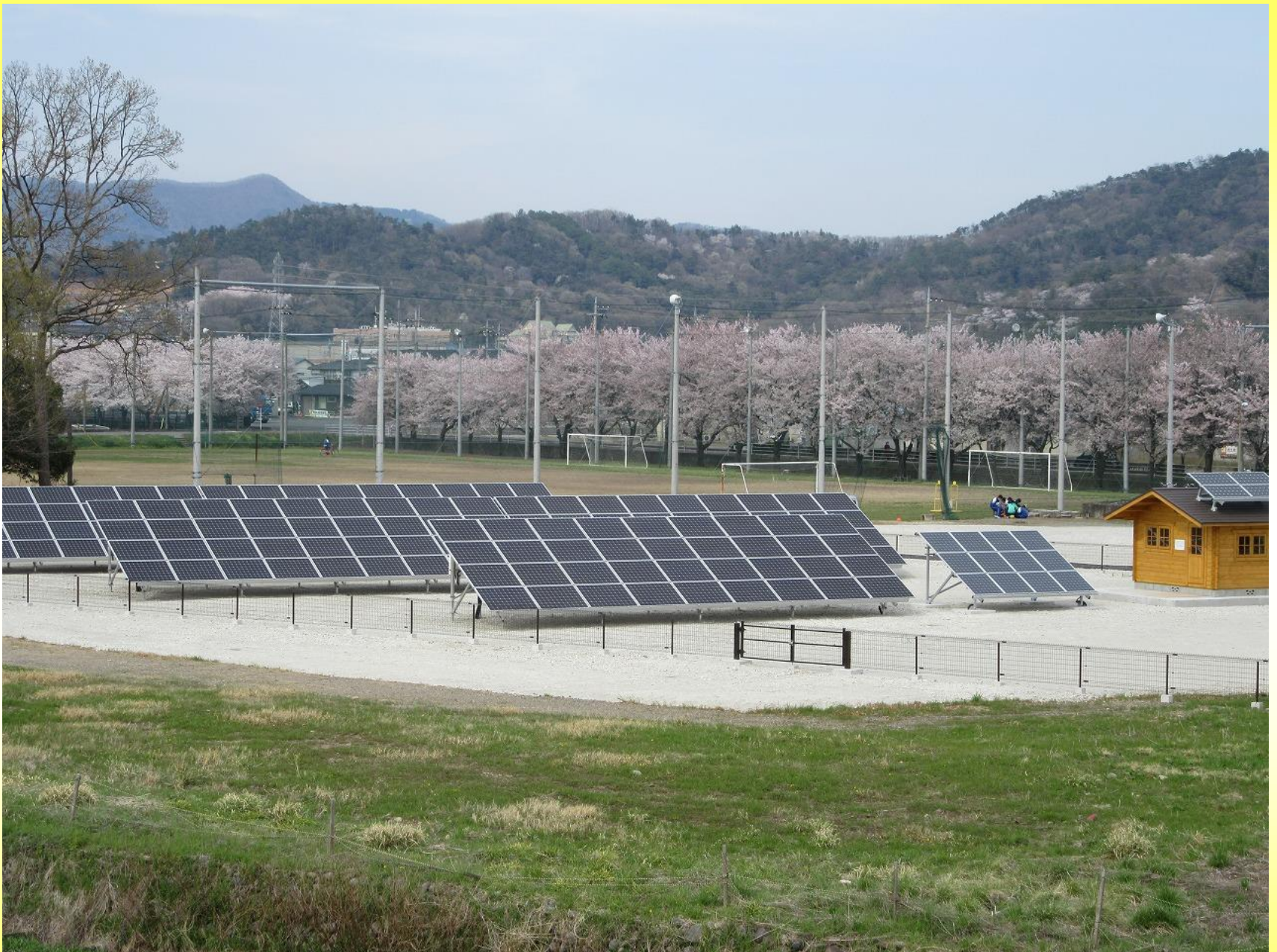
50kW PV Generation System in AU
